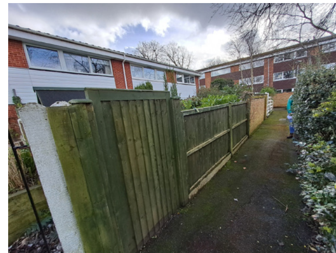
Inappropriate replacement of boundary treatments.
