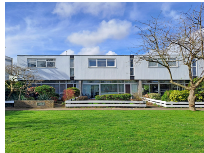
Many windows in the estate have been replaced with uPVC units as shown here at first floor level and in the central dwelling at ground floor.
