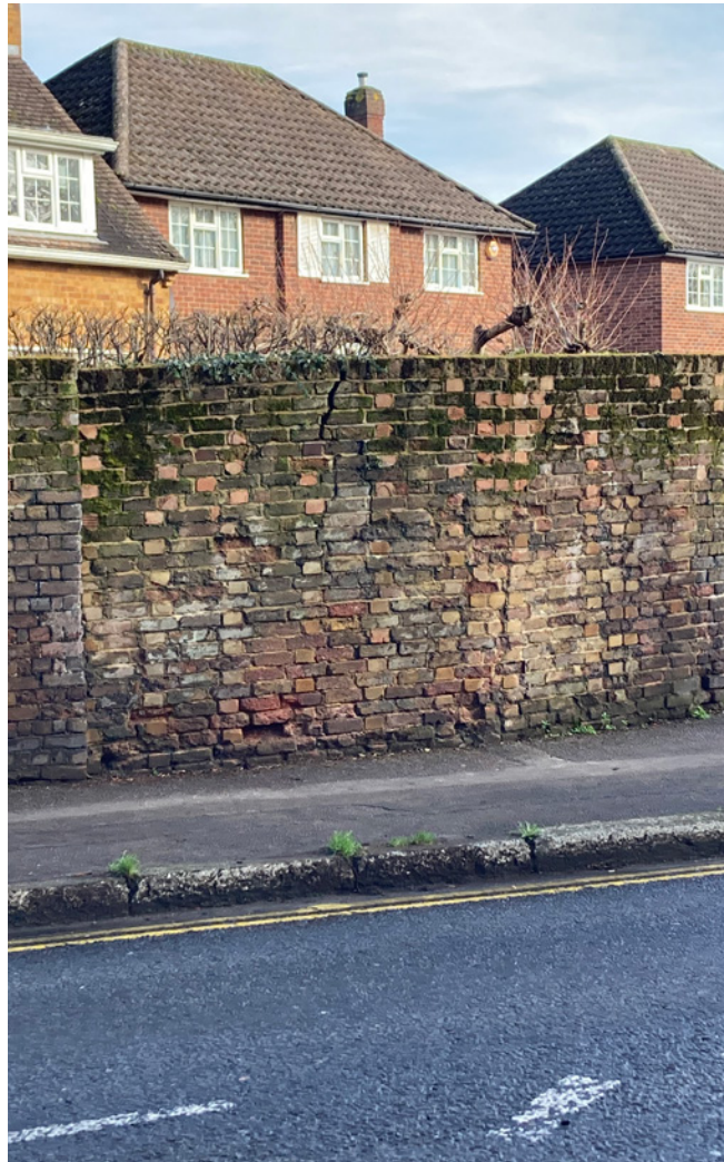
Many of the important brick boundary walls along the north side of Russell Road are in a deteriorating condition and in need of appropriate repair.
